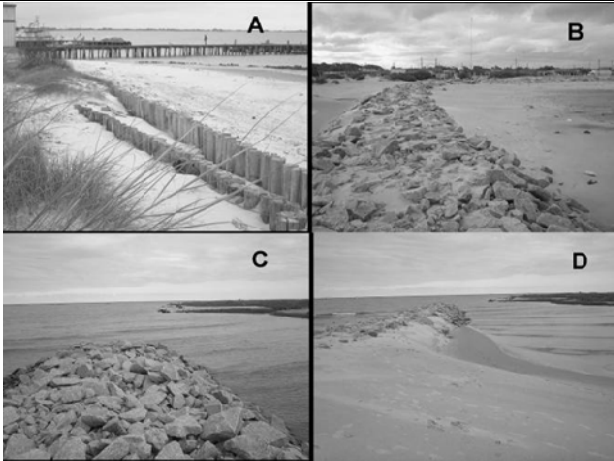
Figure 4ABCD. Initiation of jetty construction. Photos from 2006: (A) palisade made of eucalyptus trunks and (B) beach formation; Photos from 2007: (C) end of the jetty and (D) entry of the canal into the salt marsh. Water entry into the washout can be observed. SSW winds.
